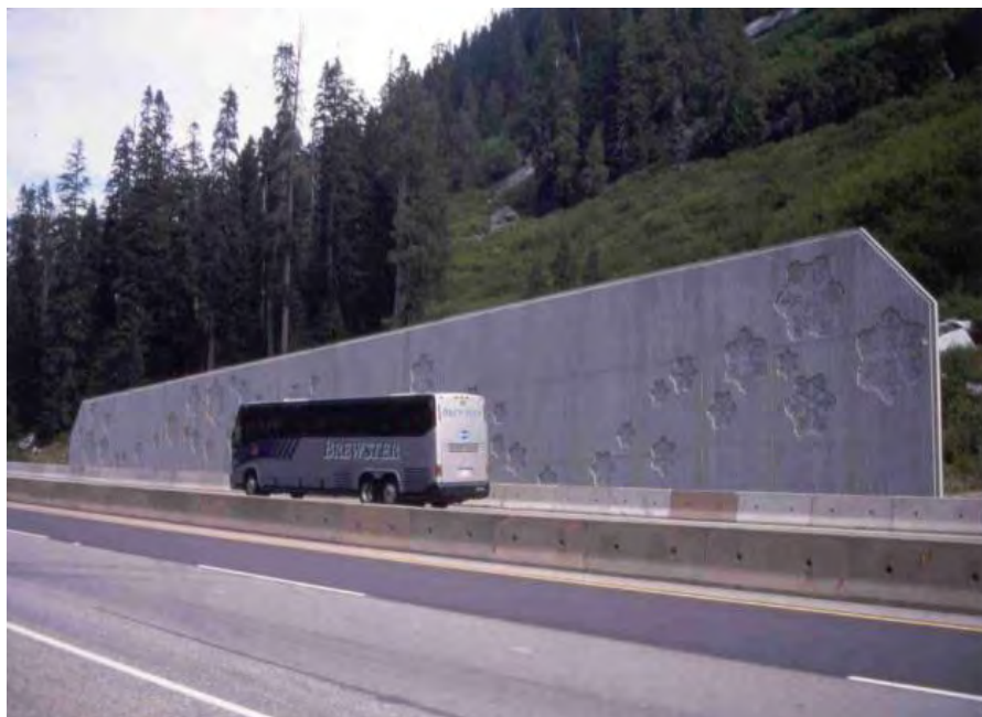
Figure 4-4: Avalanche stopping wall to stop small to medium size avalanches from impacting a highway.
