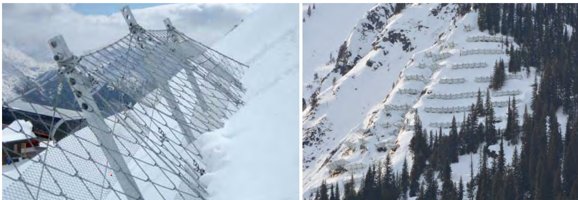
Figure 4-2: Snowpack supporting structures (i.e., flexible snow nets) in an avalanche starting zone.
